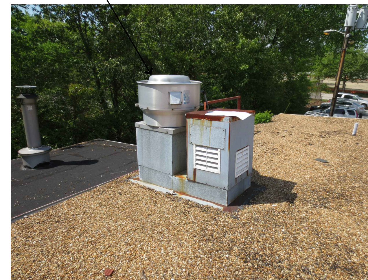
3 EXAMPLE ROOFTOP EQUIPMENT
